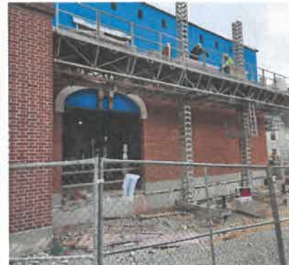
The Addition (and Sally Port Driveway) Added to the Police Station, Under Construction
